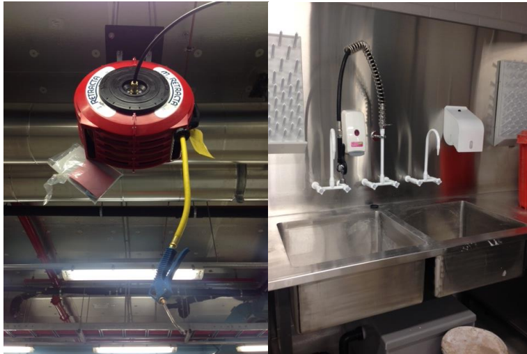
Figure 5 – Suspended air hose and sink in LG029/30
